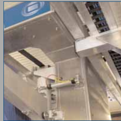
Overhead Rail System
